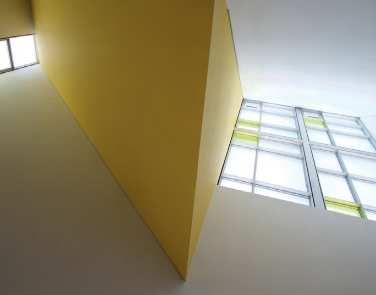
Figura 6. Lucernarios de presbiterio (2015). ©Ricardo Santonja/I+D+ART / Figure 6. Skylights of the high altar (2015). ©Ricardo Santonja / I+D+ART.
