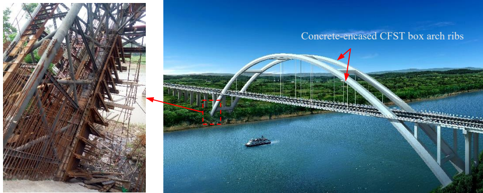
(d) A typical arch bridge with concrete-encased CFST box arch ribs in Sichuan Province.
