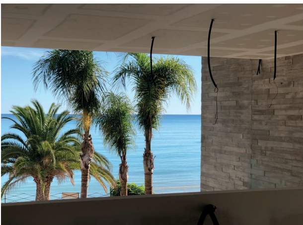
Figure 7. Details of NW and SW façade gaps. 2019. sanahuja&partners. 2019. ©Pablo Morán / Figura 7. Detalles de huecos en fachadas NO y SO. sanahuja&partners. 2019. ©Pablo Morán.
