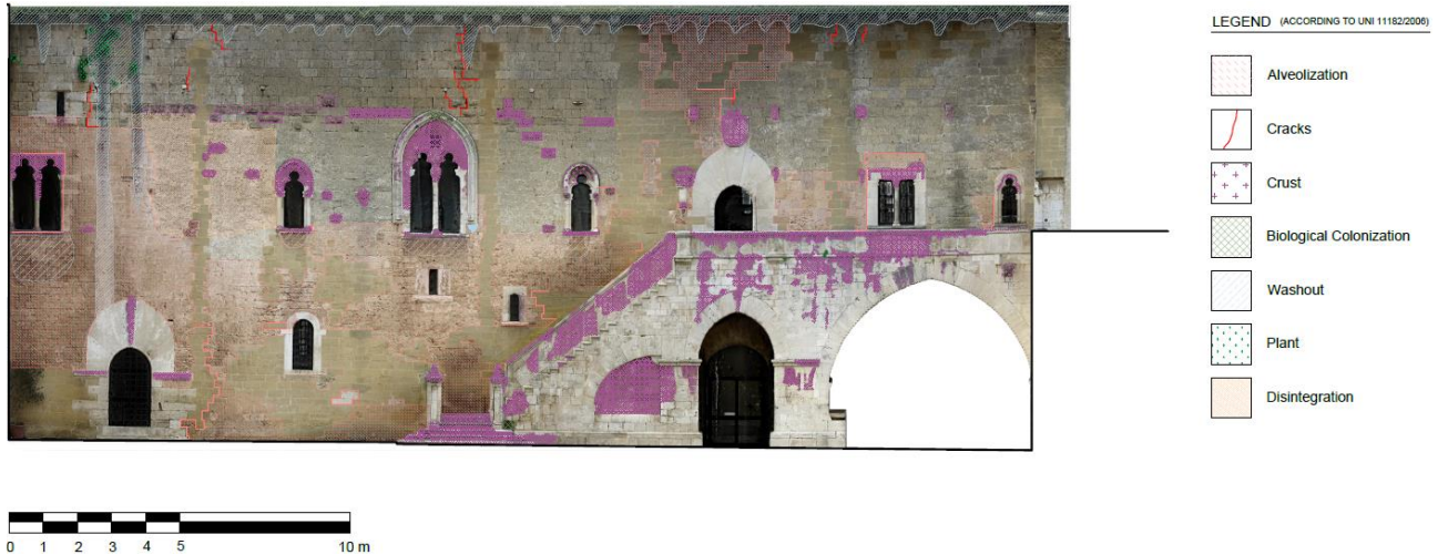
Figure 8: Performance Assessment Virtual Tour. Example of an orthophoto of the west courtyard facade, modified for decay mapping.
