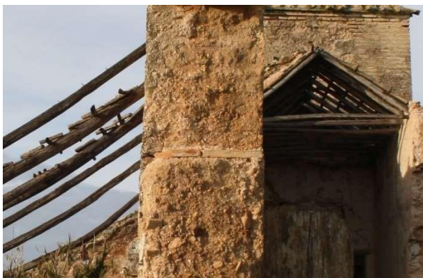
Figure 11: Detail of the rammed earth wall with mortar and a single brick course that separates the different areas at the Gallego mill in Écija. It clearly shows the thickness as two stretcher bricks.
