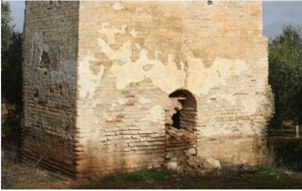
Figure 13: Opening in the counterweight tower at the Pino mill showing the wall thickness to be two stretchers.
