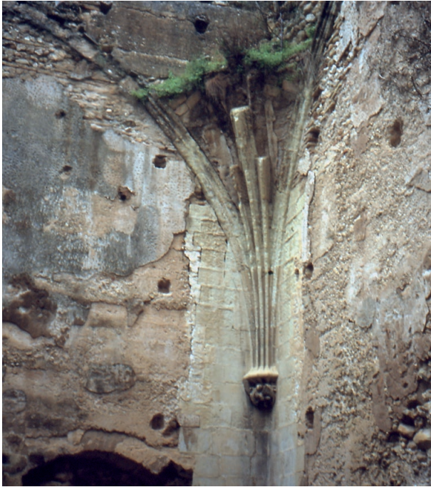
Fig. 7. Photo of one of the springs of the starred vault of the Chapterhouse in the Valldigna monastery. (Source: Capilla, Esther, 1998).
