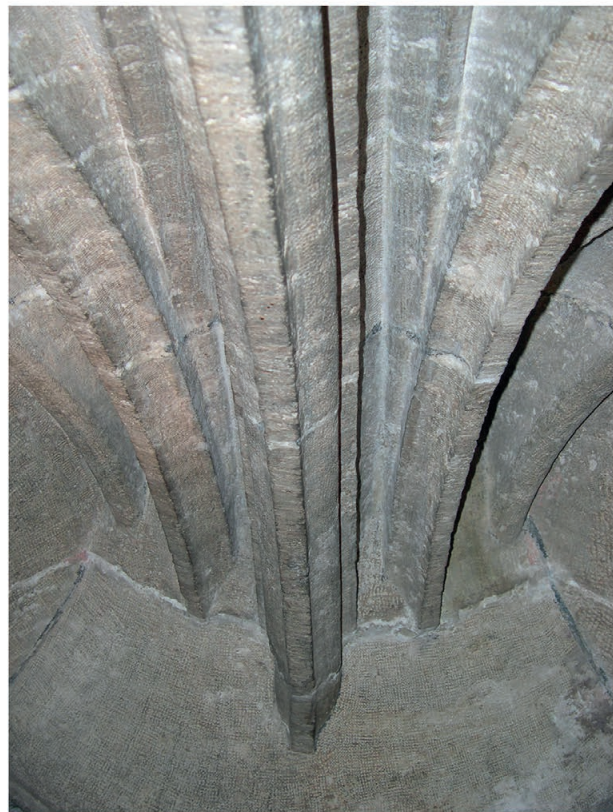
Fig. 1. Detail of the spring of the star vault of the Lonja Chapel in Valencia. You can see the corbel and the ribs that come out of it. (Source: Capilla, Esther, 2004).
