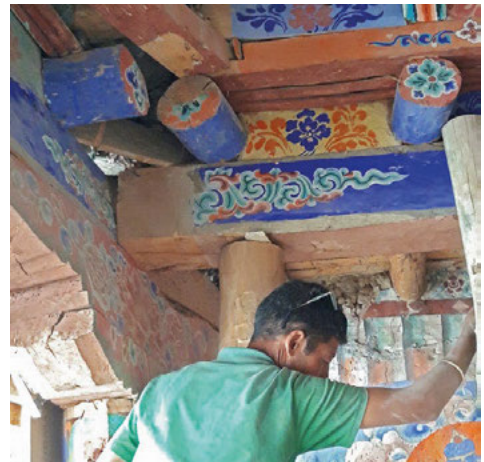
Fig. 11. One of the main beams slid 25cm outside its original position (North-eastern corner).
