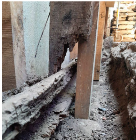
Fig. 7.a. Stone foundations and damage in bearing wooden elements in original walls (Source: Authors, 2021).
