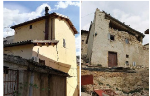
Fig. 5. Left: pounding owing to staggered roofs (Pieve Torina); right: masonry crumbling and r.c. roof collapse (Campi Alto)
