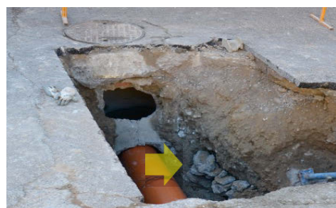
Fig. 6. Supporting the previous argument, it is especially relevant to observe in the two photographs 5 and 6, the holes or highly washed areas that appeared next to the manhole and collector (indicated with an arrow). These have been filled with rubble from the excavation itself, to later proceed to pour the sealing concrete of the connection socket of the new collector with the manhole. These two points would be connected and present a clear continuity parallel to the collector and apparently towards the lower part of the church's street.
