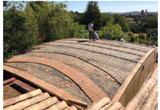
Fig. 5. Salva and Jesus Gomis working at the construction of an inclined sail-vault reinforced with ribs. This tile-vault has a 7:30 m span and a rise of 25 cm on the back and 12 cm on the front. (Source: Vitti)
