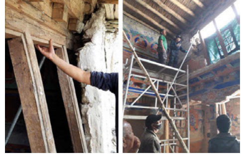
Fig. 10. Tilted wooden opening on the first floor (left); covering the paintings with a protective cloth near the wooden window (right).
