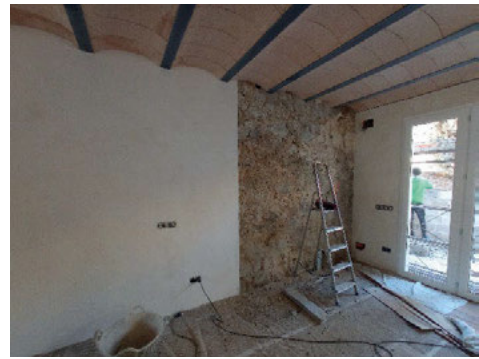
Fig. 6. Cover of interior stone walls, made by calcic lime mortar, leaving parts of uncovered walls (Source: Li Puma, 2021)
