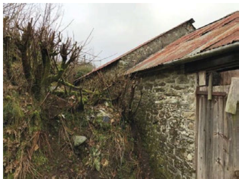
Fig. 7. Build-up of spoil and tree growth against south wall prior to excavation (Source: Jonathan Rhind Architects, 2019).
