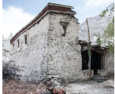
Fig. 4. Main entrance and porch. The temple started to shift from this corner at the base of the walls (North-east).
