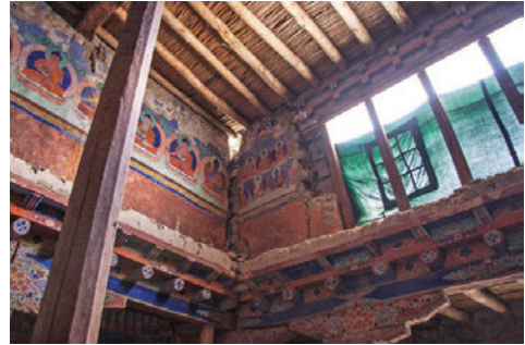
Fig. 7. The severely damaged, tilted, and detached walls on the first floor of the temple's chamber (North-west corner).
