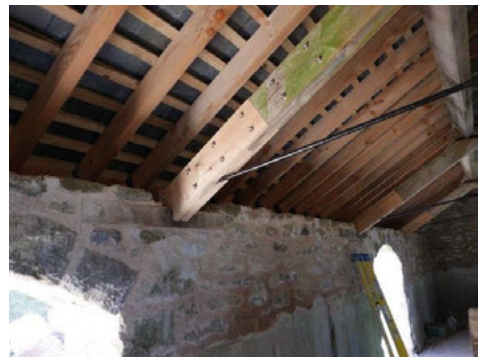
Fig. 12. Fitch plate repairs to feet of principal rafters at Great Cator (Source: White ,2021).
