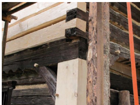
Fig. 3. Watermill No. 2 (82) and new members instead of damaged ones, the replacement requires additional supports and load securing, e. g. by carrying straps/webbing on the right, Zubrnice Rural Reservation, Ústí nad Labem District, Ústí nad Labem Region © Martin Cernansky, 2015, NHI
