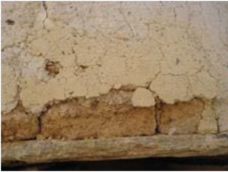
d) Adobe and earth mortar
