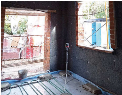
Fig. 8. Insulating by recycled cotton and radiant heat, kitchen area (Source: Li Puma, 2021)
