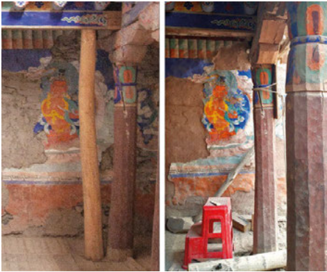
Fig. 19. Tilted structure with prop (left). The unpainted part of the beam marks the extent of the rotation of the column. The structure after it had been straightened (right).
