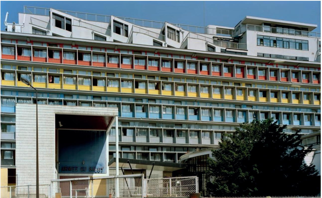
Figure 4 | Front façade oriented to the south after retrofitting. Cité de Refuge , Paris. © Olivier Martin-Gambier 2005© FLC/ADAGP.
