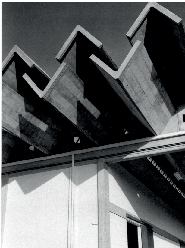
Figure 3 | Manifattura Ceramica Pozzi Factory, Sparanise, Caserta, 1960-64. Architects Luigi Figini & Gino Pollini. Detail of the prefabricated structural system of the paint compartment. (Photo: Carlo Orsi. Museum of Modern and Contemporary Art of Trento and Rovereto, Italy - MART, Archive of the XXth Century, Archive Luigi Figini e Gino Pollini).
