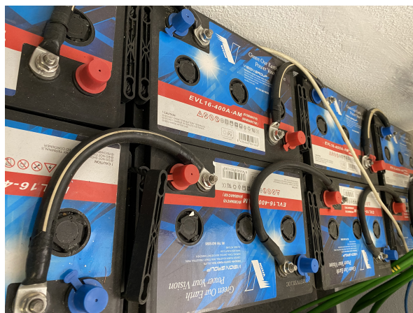
Figure A.1: Battery bank.
