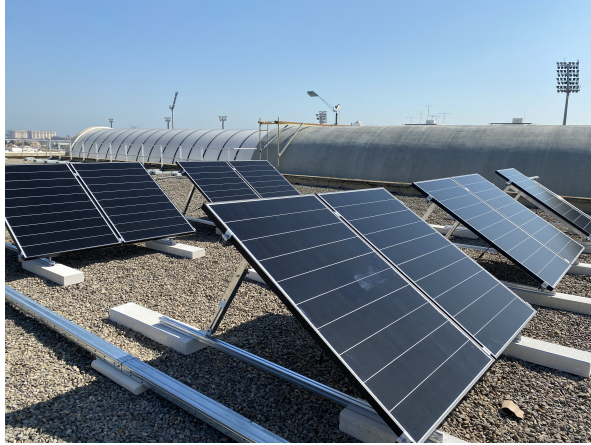
Figure A.3: PV panels.
