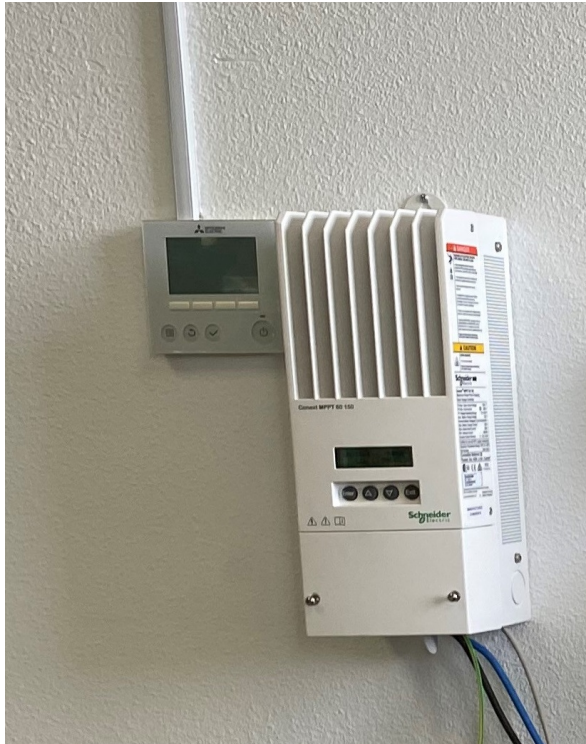
Figure A.2: Charge controller.
