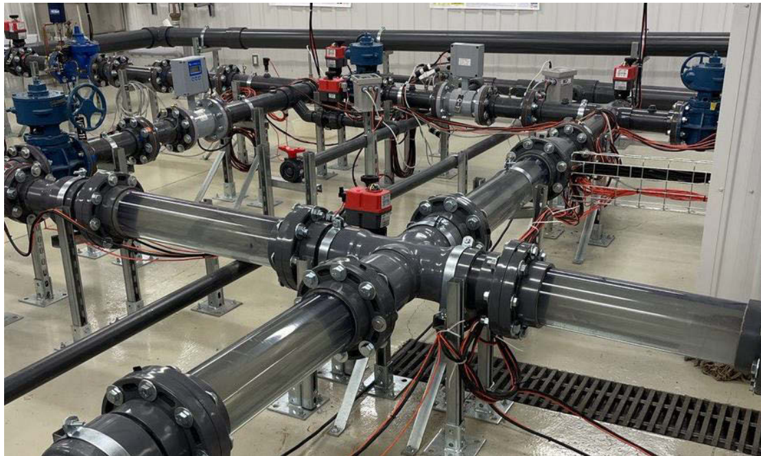
Figure 2. 150-mm cross junction used in mini water distribution network laboratory of INRS
