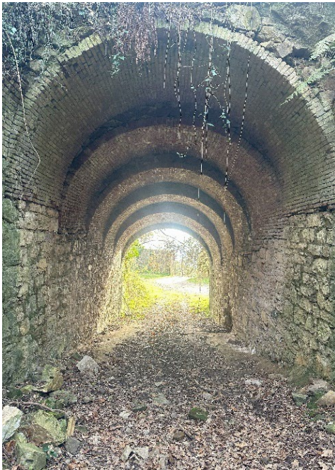
Fig. 2- The entrance passage under the Traversone . View of the lower court yard (Marinara, 2023).
