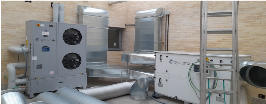
Fig. 3 – Aerothermal and heat recovery equipment.
