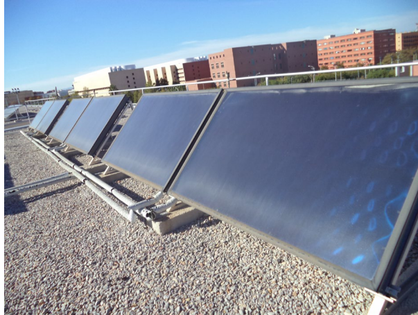
Fig. 2 – Solar Thermal Installation
