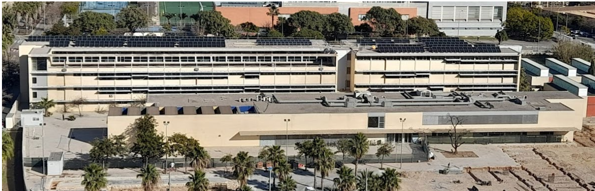
Fig. 4 – Current photovoltaic installation
