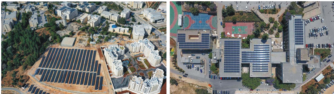
Fig. 1 – Solar PV plants at Birzeit University (1.7 MW)
