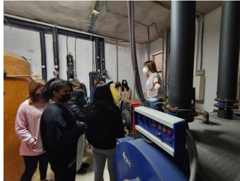
Fig. 2 – Group of Student visiting the boiler room of their centre during a thermal tour
