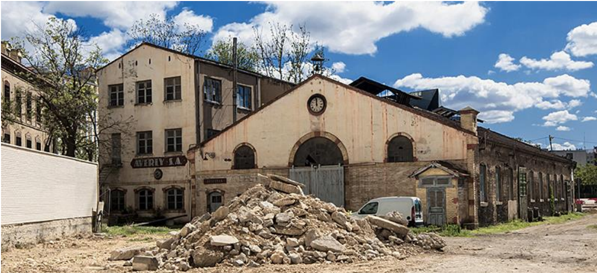
Figure 8. Current view of the Avery foundry among the rubble and the new block of flats under construction. Author: Antonio Duaso Clusa.
