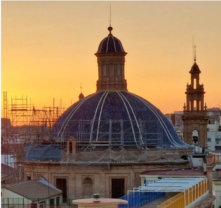
Figure 2. The dome of the Church of the Pious Schools of Valencia during its restoration in 2024. Source: Cortés, L. (2024)
