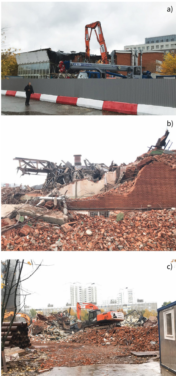
Figure 6a | Initial stage and glass façade destruction (Author, 2019).
