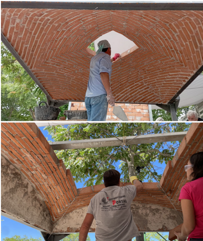
Figure 1. Vaults under construction, above by Andrés Flores, below by Máximo Portal. (Image by the authors).
