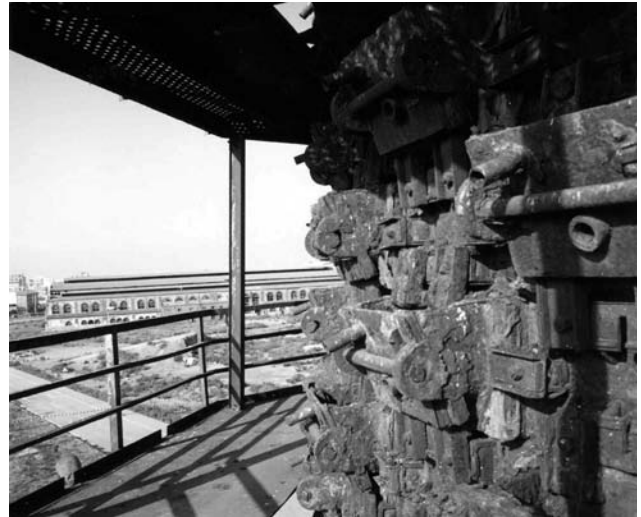
Figure 2. View of one of the barrel platforms. In the foreground, the cooling unit is covered in rust
