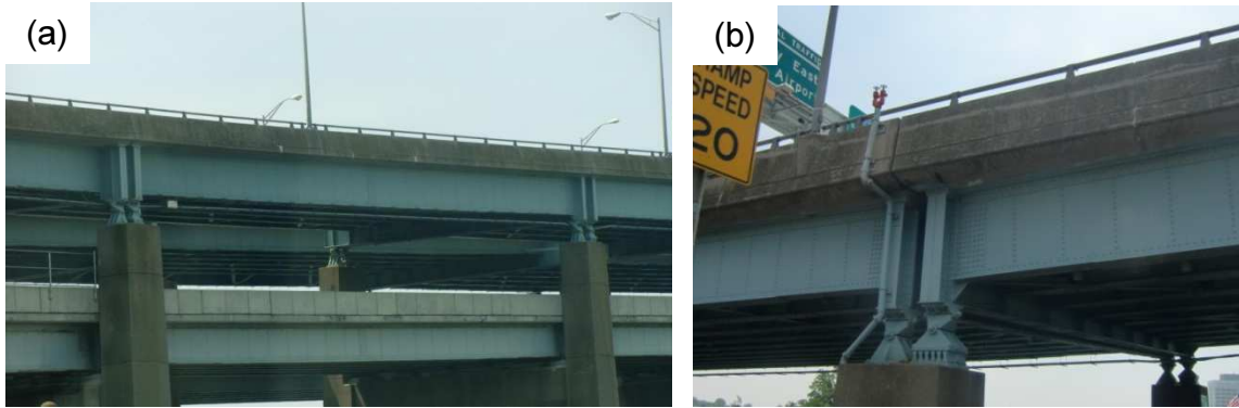
Figure 1. Typical simply supported steel girder bridge (approaches to the Verazzano Narrows Bridge, USA): (a) general view, (b) detail of the bearings.
