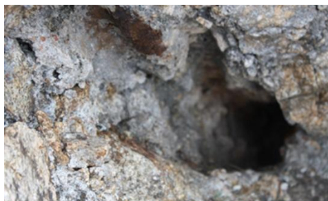
Fig. 7 -One- collapse piece Sponsaglia tower's
